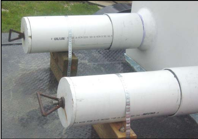
Pipes on back of tank
