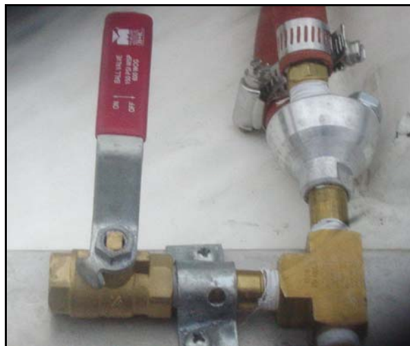
Ball valve on oxygen supply line in the closed position
