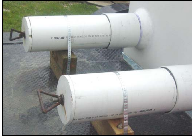
Release tubes on back of tank
