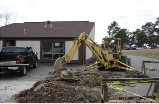
City Water Leak In the Middle of the Parking Lot
