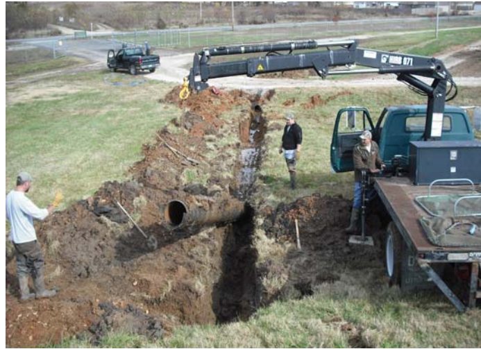
Tom removes old pipe with boom loader as Heath and Clarence directs.
